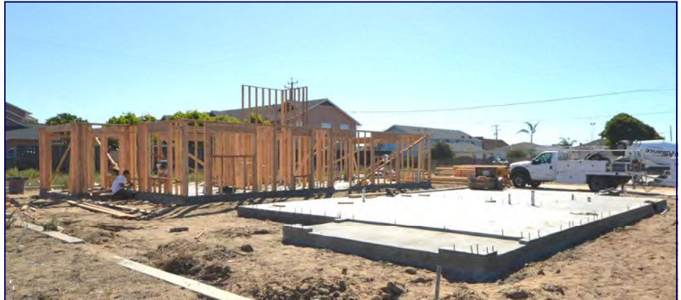
Construction is underway at Peoples' Oceano self-help housing project. The HTF provided a $600,000 construction loan for the six families to build their own homes.
