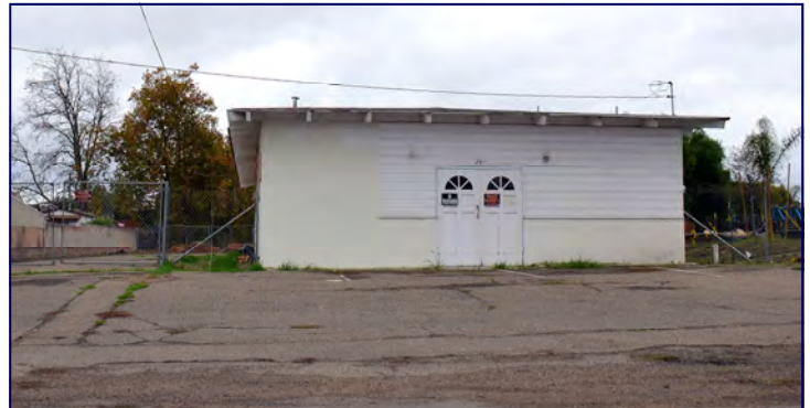
Vacant building on Thompson Avenue in Nipomo that will be rehabilitated and converted into Head Start classrooms.
