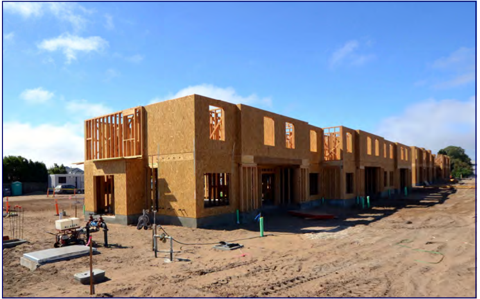
Construction is progressing at Peoples' Courtland Street Apartments in Arroyo Grande. The HTF provided part of the construction financing for these 36 affordable rental homes. Construction should be completed by the fall of 2014.
